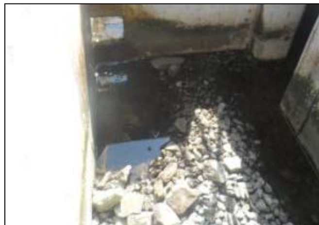
Fig. 12: Water pools created by concrete metal
