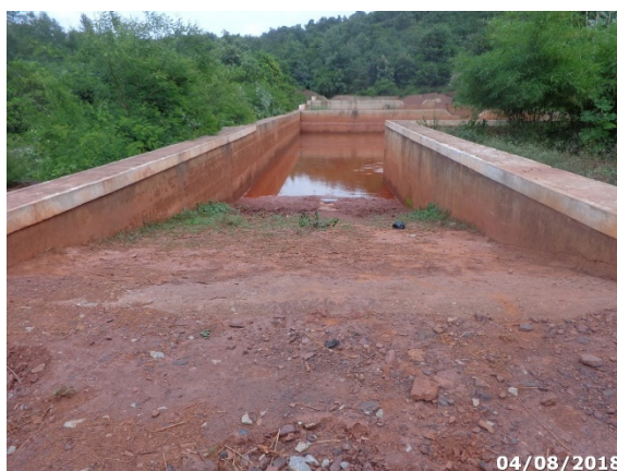
Figure 7 Settling tank for retention of drain off water.
